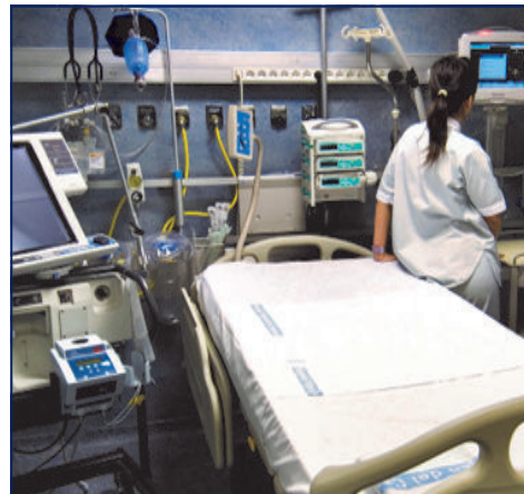
Inov8 AD units in hospital theatres.
